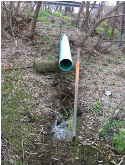
This outfall, though in poor condition because it is cantilevered, provides a good opportunity for a clean catch of its discharge.
